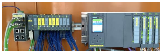
neue Siemens CPU 1517F-3 PN/DP
